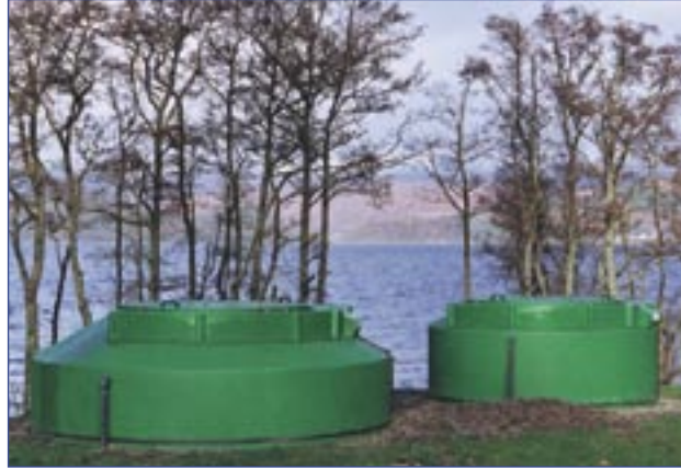
Two installed Aquapoint Bioclere units.
